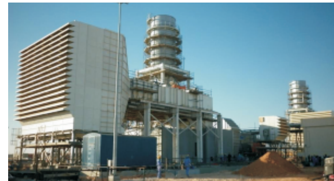
2xFrame 9E GTG order under execution at PDO Amal site in Oman
