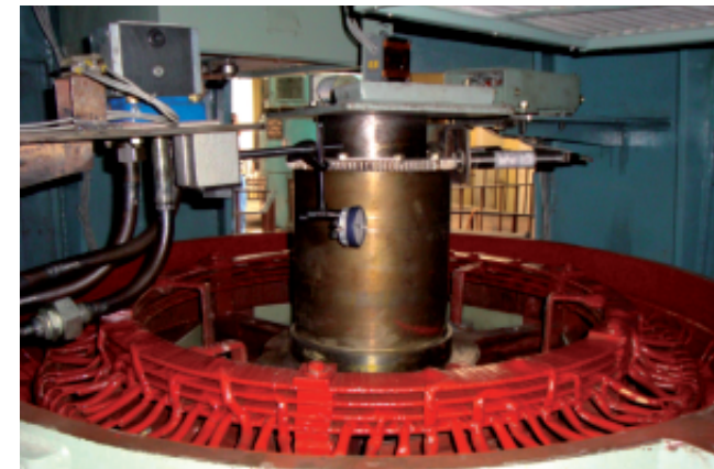
Brushless Exciter developed at BHEL's R&D Centre installed at Devighat HEP, Nepal
