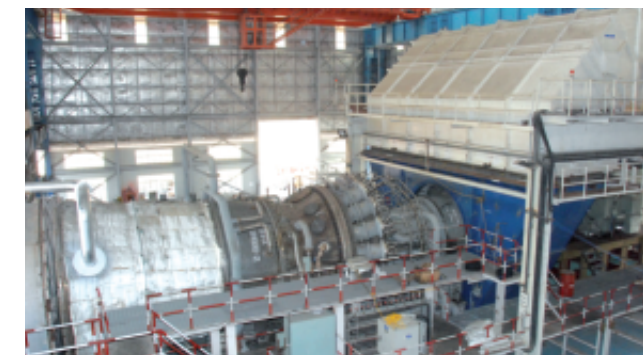
India's first indigenously built 9FA (250 MW ISO) Gas Turbine set manufactured by BHEL
