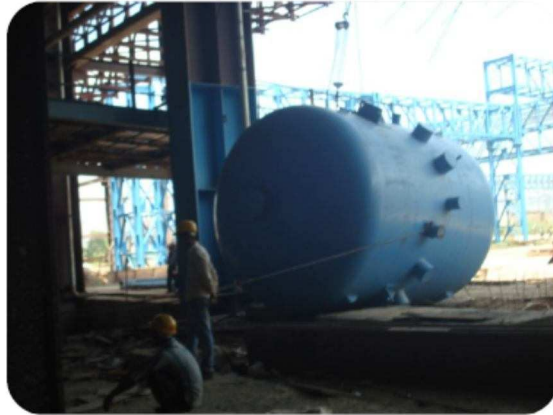
Flash tank being brought from A-row side
