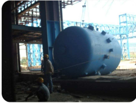
Flash tank being brought from A-row side
